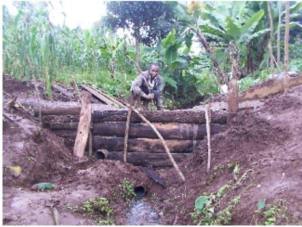
Shuttering in place during application of cement layer to seal the weir
